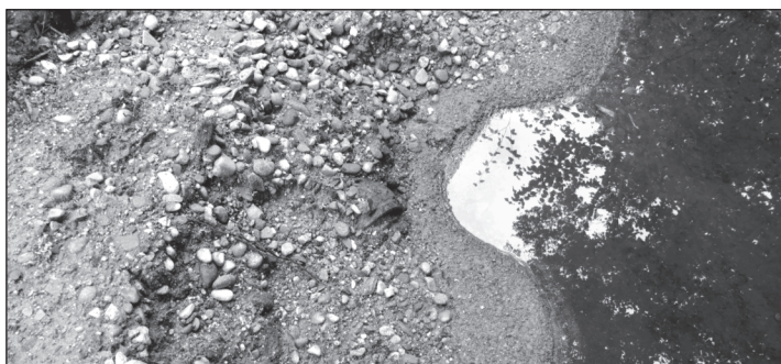
A remnants of a very old, small diameter iron pipe on Jenkins Road that did not provide proper drainage.
